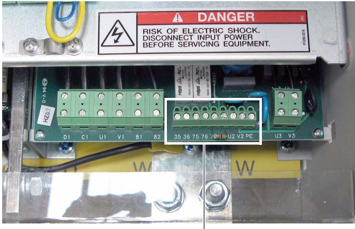
Figure 39 - 230V/460C AC Input Frame C Relay and Thermistor/Thermal Switch Terminal Block Locations
